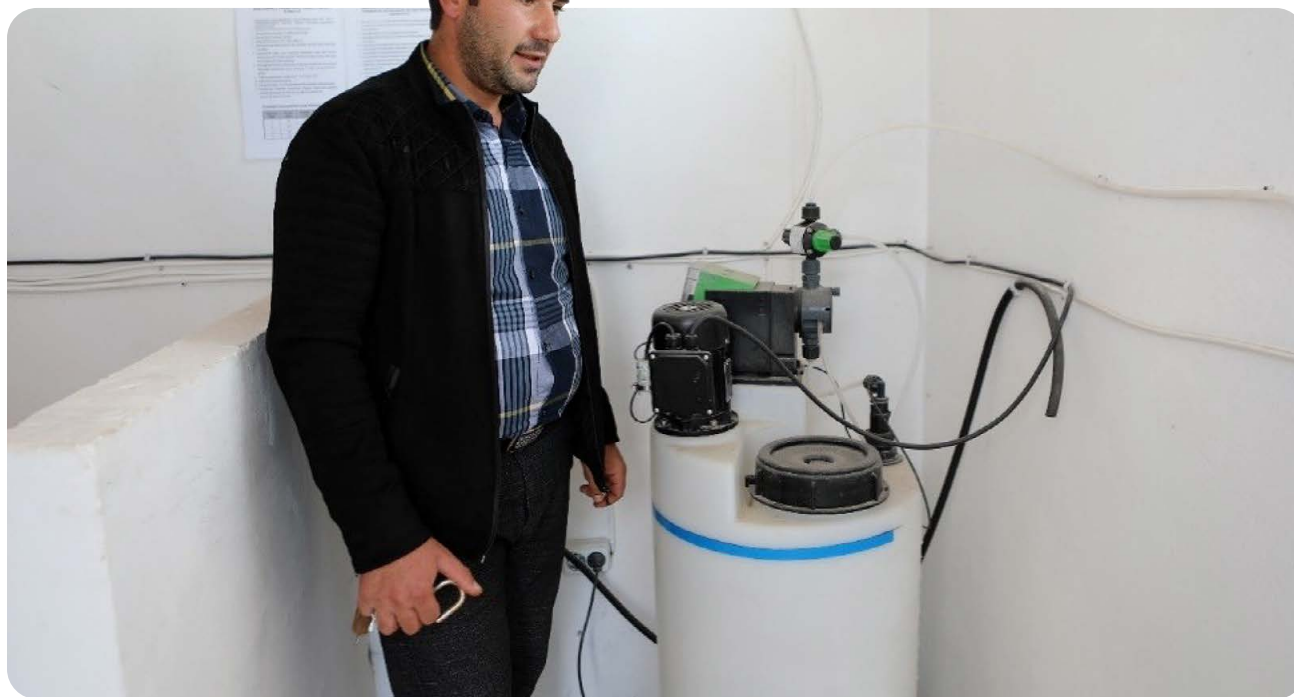
Chlorination station equipment installed in Basen. Hayk Mnatsyan (pictured) is the village administration specialist for the station ©Sustainable Caucasus
