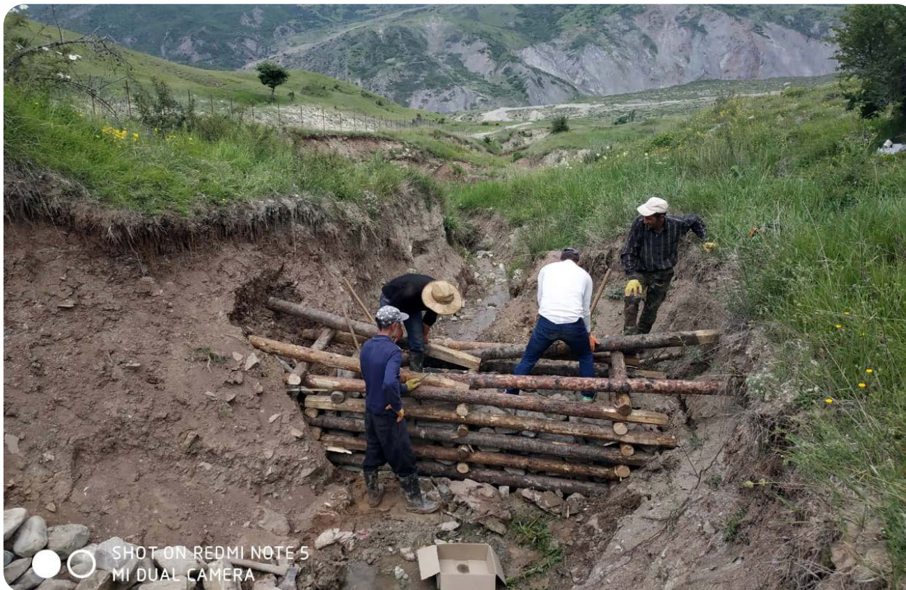
A wooden check dam under construction in the pasture area of the village Ehen, Azerbaijan ©Sustainable Caucasus
