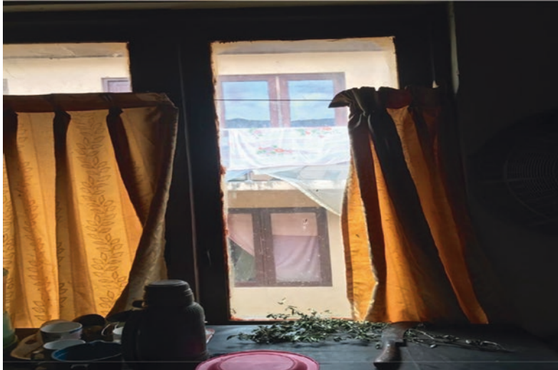
Image 3 Unsafe windows. Source By the researcher, 2023
