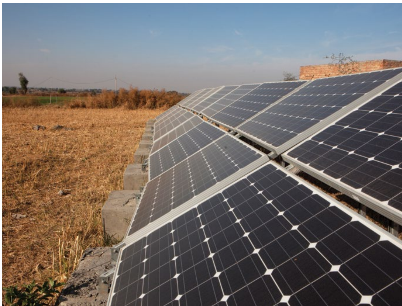
SOLAR POWERED WATER PUMPING SYSTEM, TALAGANG, PAKISTAN.
